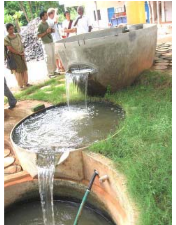
Grey Water Treatment
